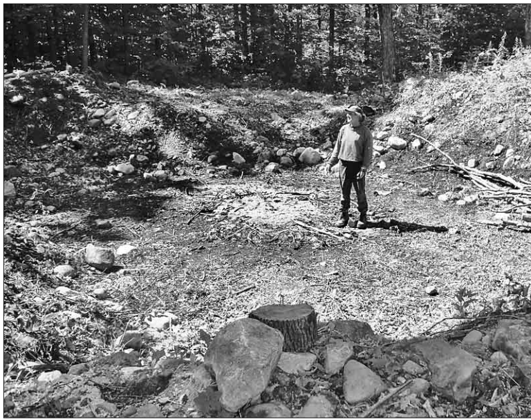
Clayton Trudeau stands inside the large hollowed-out area that will be developed into a huge root cellar, or sanjgon, in Wikwemikong.
